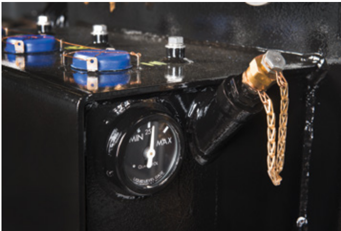
Switch-box liquid-level gauge and filling provision
